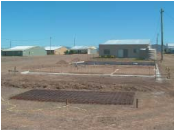
Building gets underway once more at Watts. An early shot of Derek Robinson's Airchalet footings, just poured.
